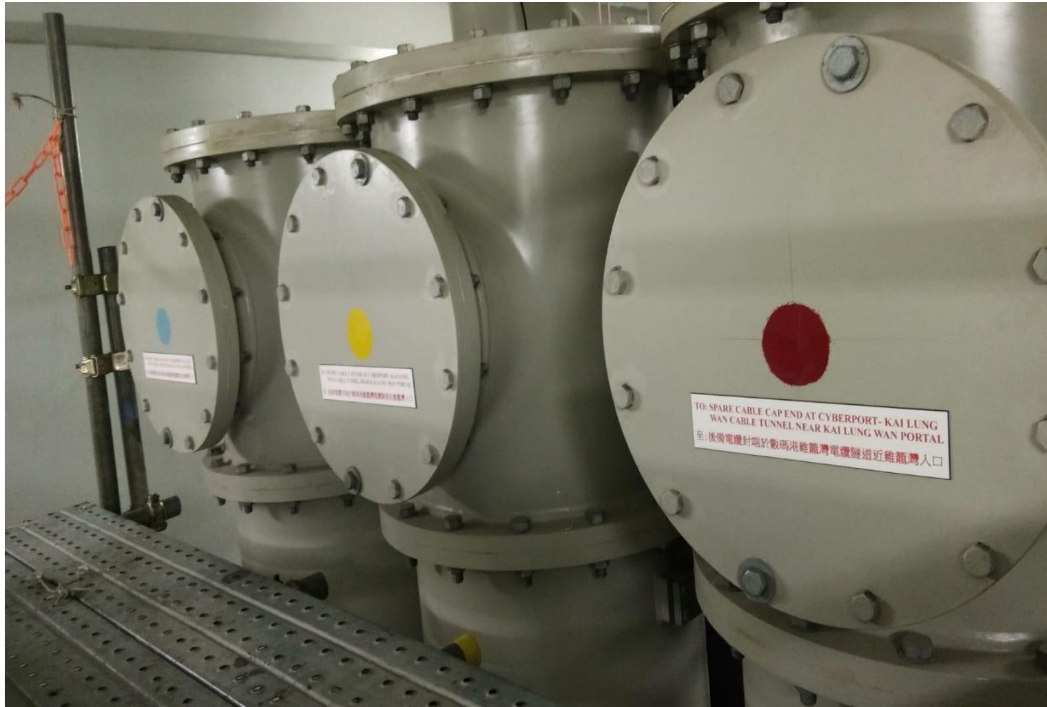
Figure 5. New Labels with Additional Information on Cable Connection Tank at CPX
