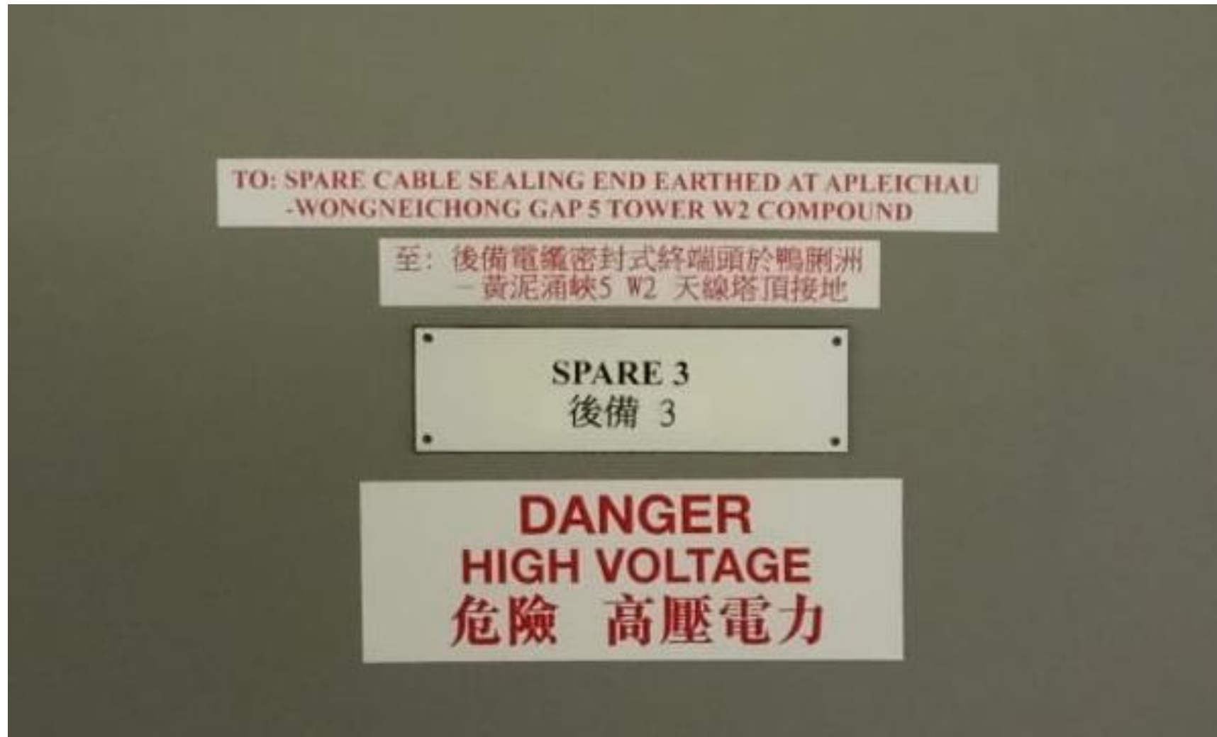
Figure 7. New Label on the Cable Connection Tank at Apleichau 132-kV Switching Station
